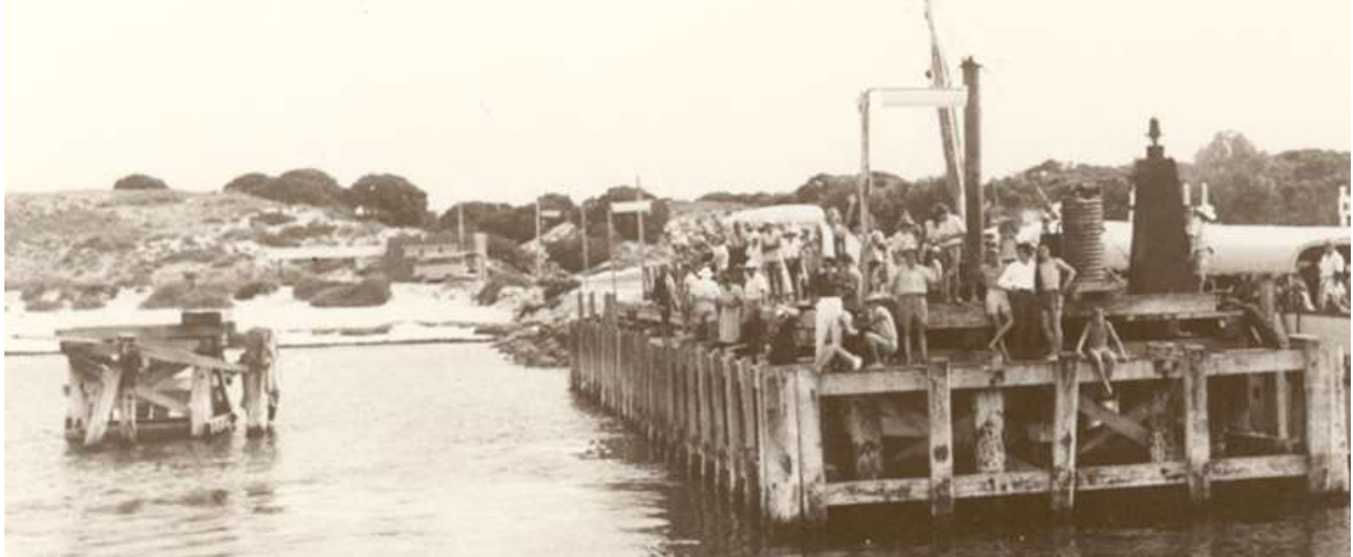
The jetty extended and the dolphin nearing completion. Construction had to be scheduled to avoid interference with ferry arrivals and departures.
